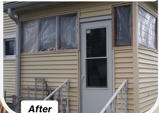
Anna's door couldn't close fully, causing safety concerns and energy loss. A new door gave her peace of mind.
